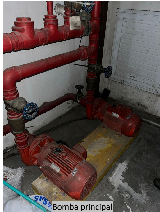
Figura 20 - Bomba principal e bomba reserva
